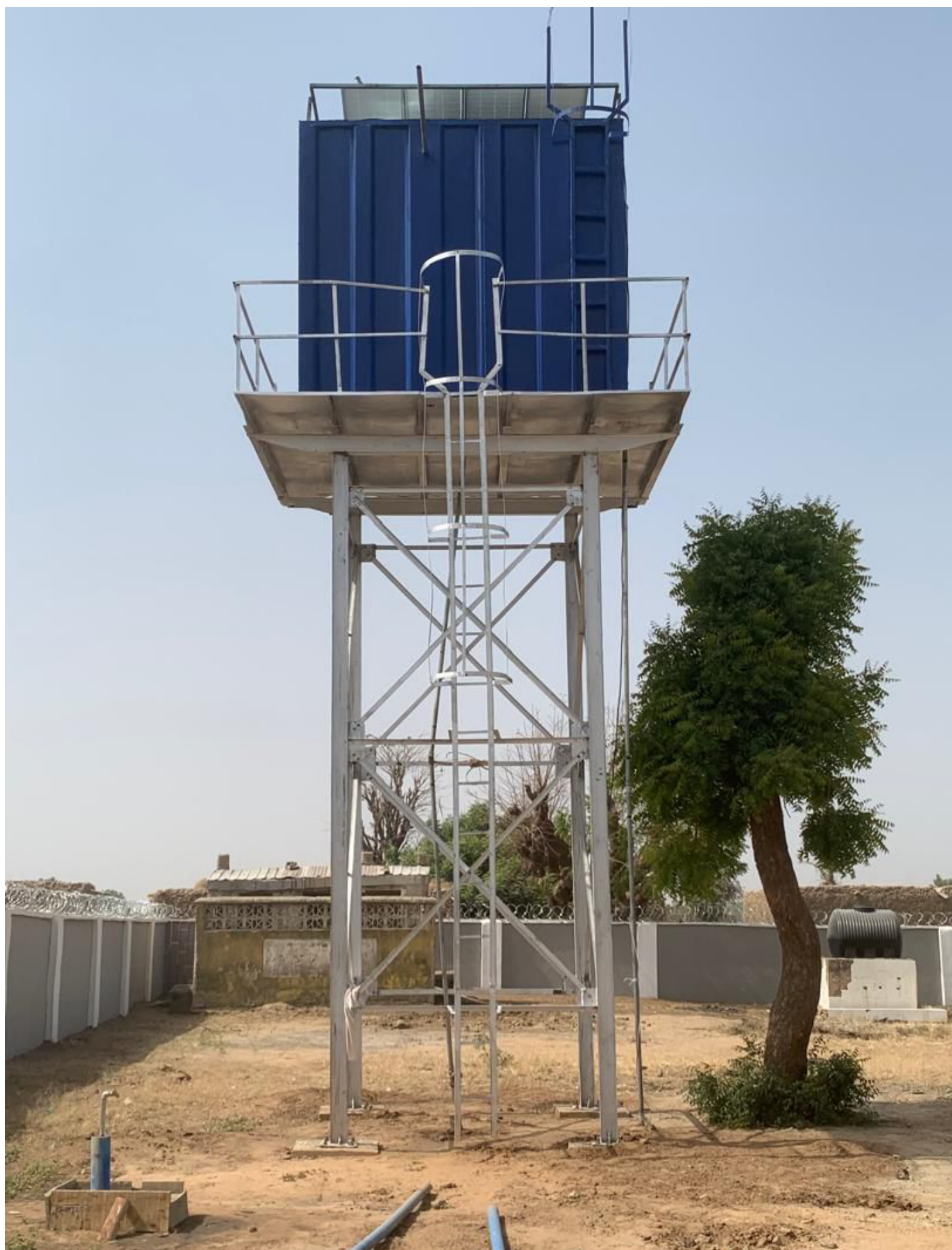
Solar water scheme at Ayan BHC
